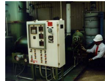
Checking vapor flow rates
